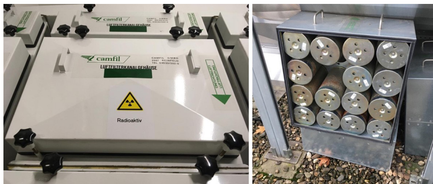
Figure 6: HVAC covering (left) and filter (right) on the building roof
